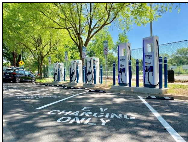
Example pull-in EV charging stations.
