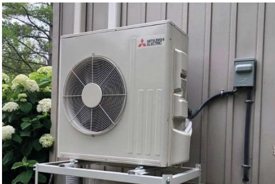
Example of typical heat pump install
